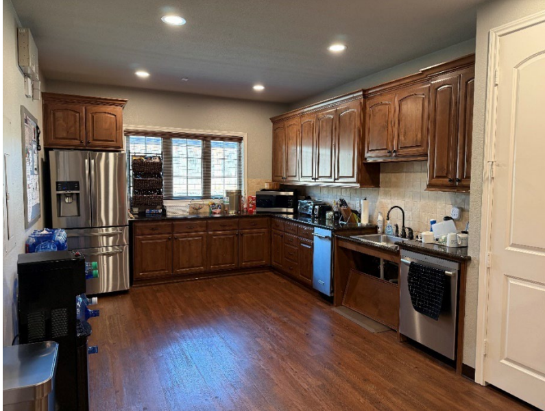
Kitchen in break room does not have a minimum 30" wide section of counter space at 34" max above floor as required by TAS.
