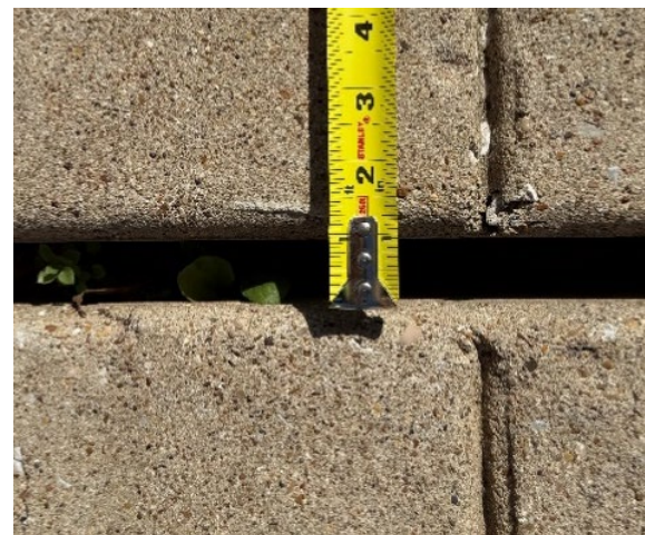
Gap in sidewalk is 1" (above); larger than the \frac{1}{2} " maximum allowed by TAS (below).
