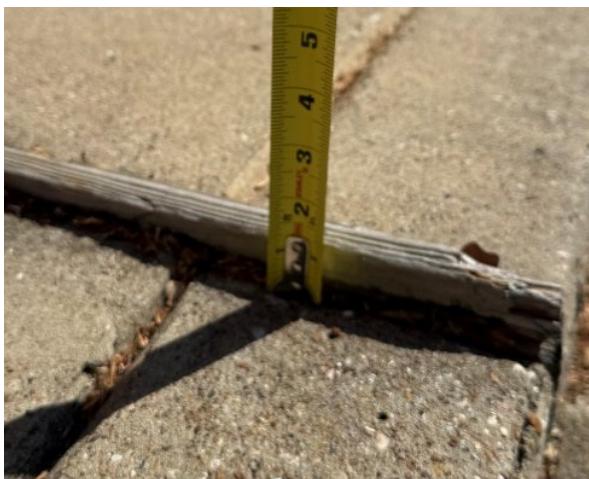
Wood extends up from walking surface 1" (above); more than the \frac{1}{4} " maximum allowed by TAS (below).
