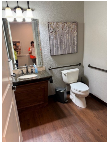
Required toilet clearance space is obstructed by vanity in back bathroom. Vanity's knee and toe clearances are below the minimum amount required.
